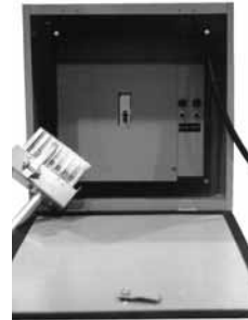
Breaker Test Cabinet
