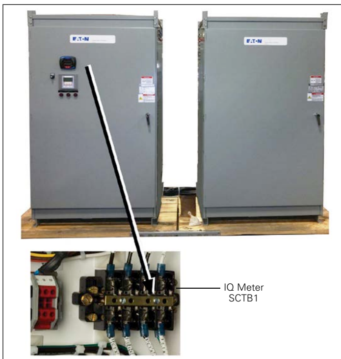
Figure 7. Current transformer shorting block for IQ Meter
