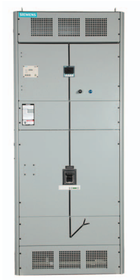
Switchboard with Sm@rt DAS
