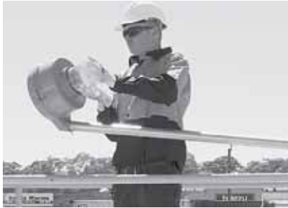
Safe and easy access to luminaire for inspection and regular maintenance
