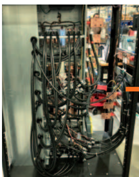
Cabinet with cables
